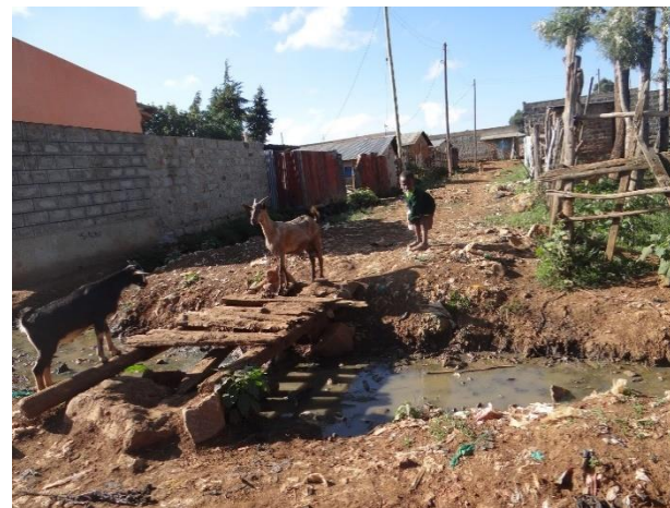
Plate 6: Blocked drain channel along Uganda Road
